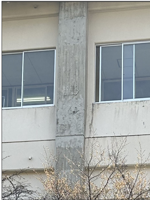
補修箇所①
